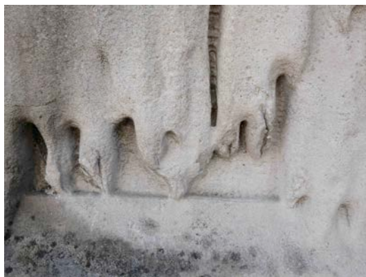
Fig 16: example of decay to Portland stone detail
