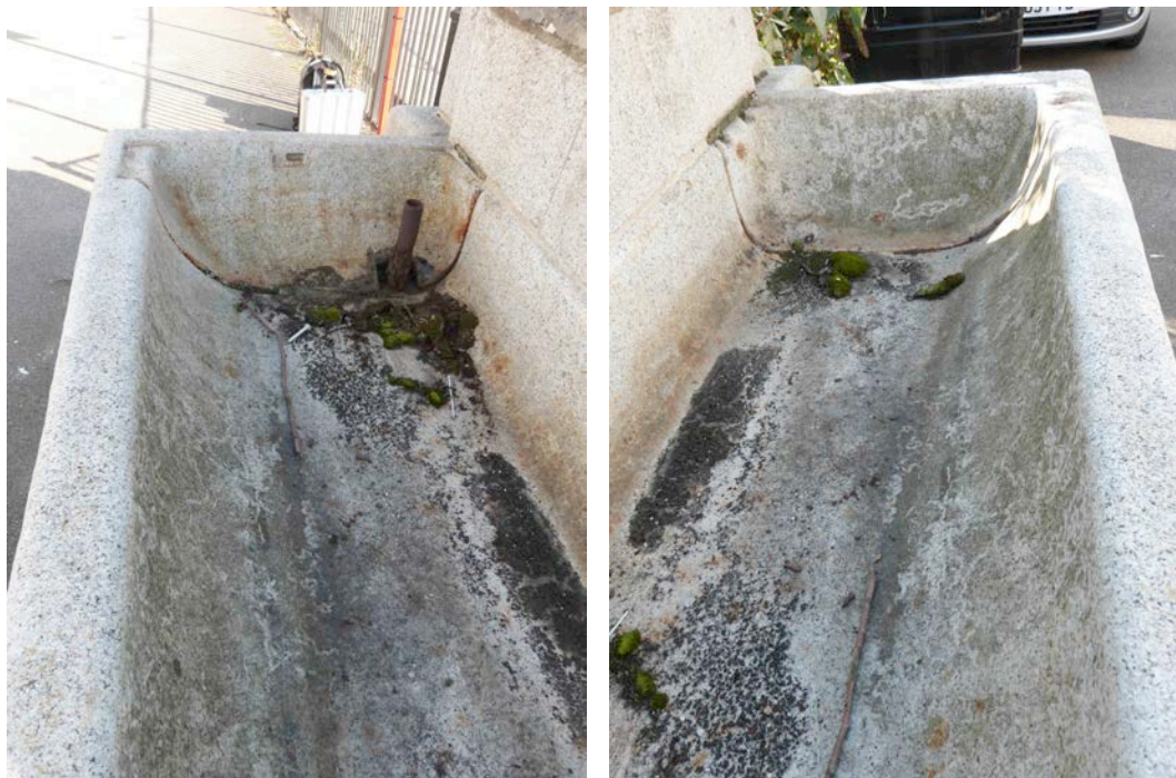
Figs 9 and 10: view of interior of main trough from the south and north
