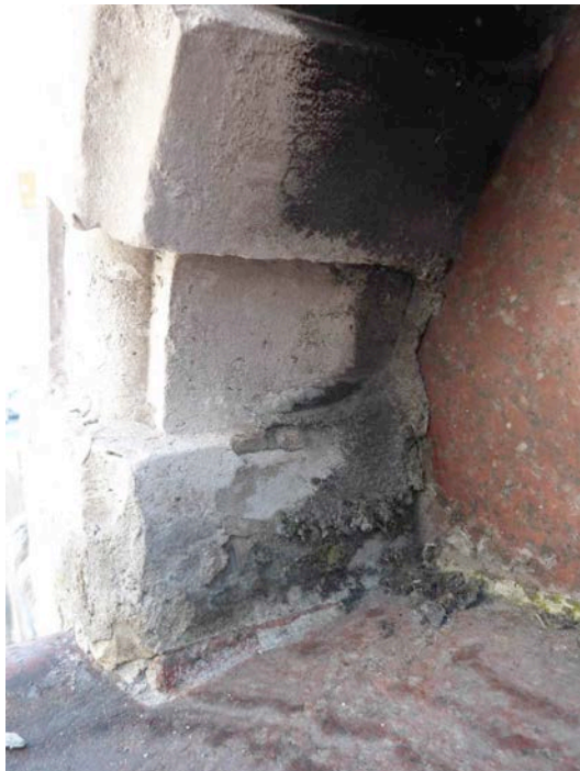
Fig 27: interior of arch (north) showing sulphation
