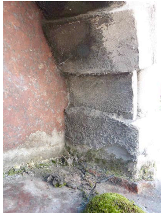
Fig 28: interior of arch (south) with sulphation
