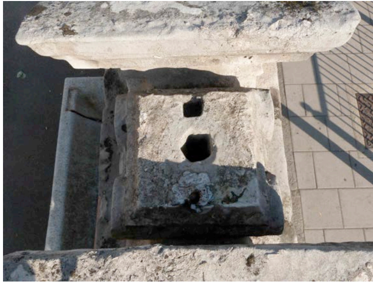
Fig 36: top of plinth of pediment showing old fixings and holes that may have been associated with lighting
