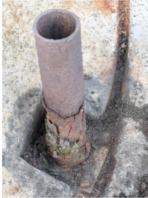
Fig 11: corroded pipe and flange plate
