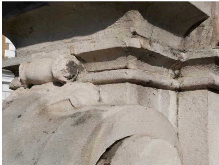
Fig 30: cracks and repair to applied section of cornice on east elevation
