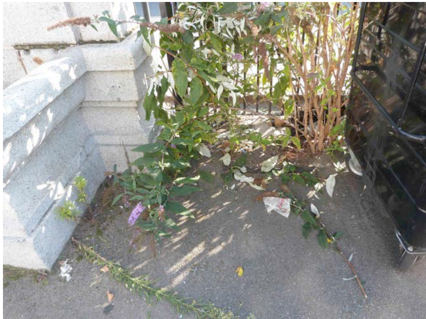
Fig 7: manhole to the south of the fountain (obscured by Buddleia bush) where water supply is accessed
