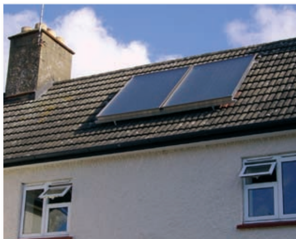
Solar water heating panels
