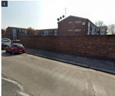
View looking east along Lansdowne Road showing the existing brick boundary wall
